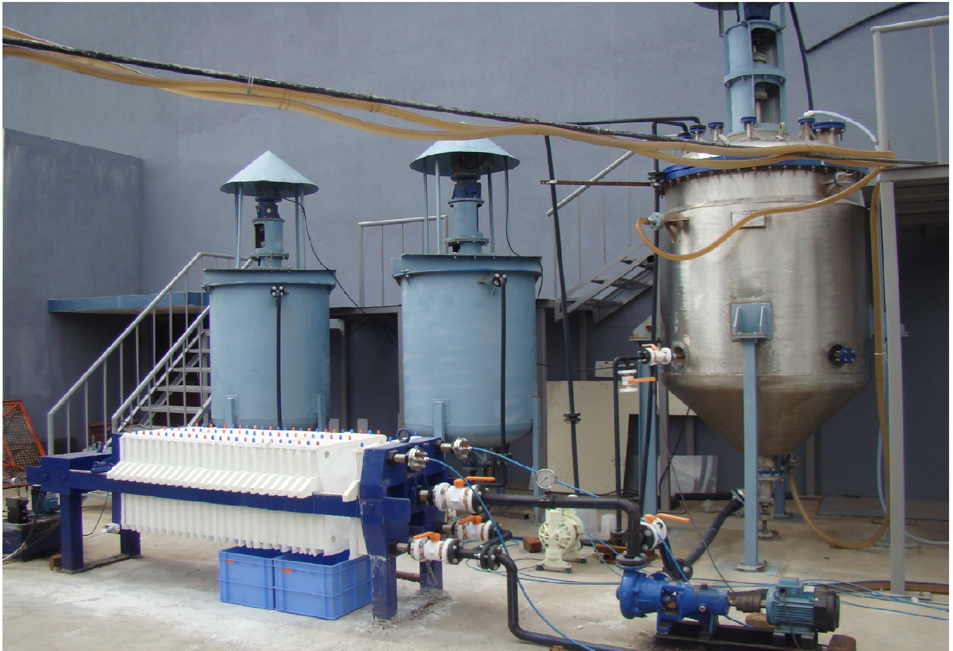
Effluent Treatment Plant for used EP Solution
